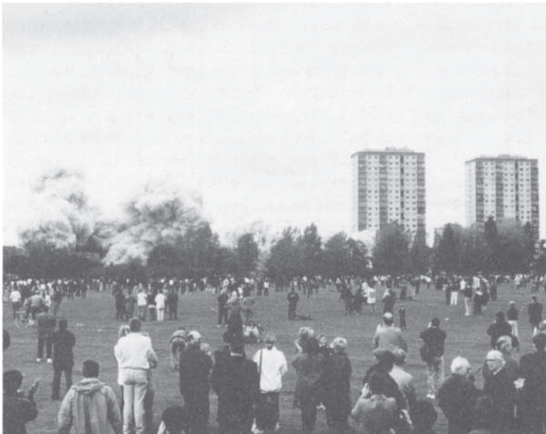
Plate 28.1 Tower block demolition, Clapton Park Estate, Hackney, London. Only one tower block remains, the rest having been demolished to make space to build new homes for rent.
